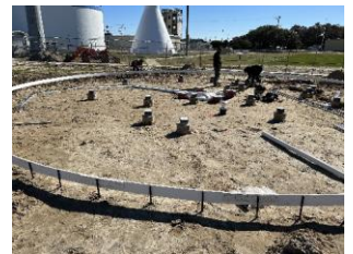
Above, pipes lead from building to Splash Pad features.
